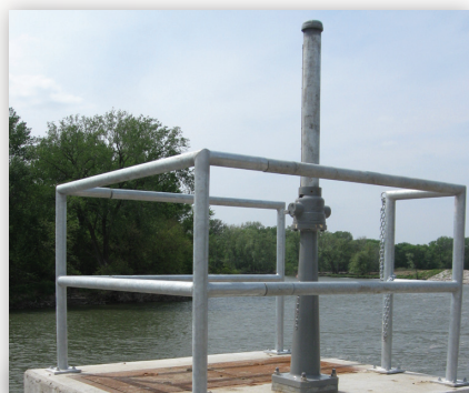
New gate wells along the Birdland Levee will better withstand future floods.
