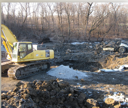
Major excavation was necessary before Story could properly pour new concrete for the Birdland Levee.
