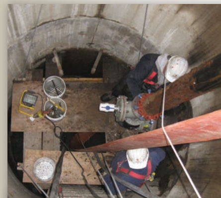
Crews worked 20 feet under ground in Iowa winter, but the temperatures stayed around 50 degrees.
